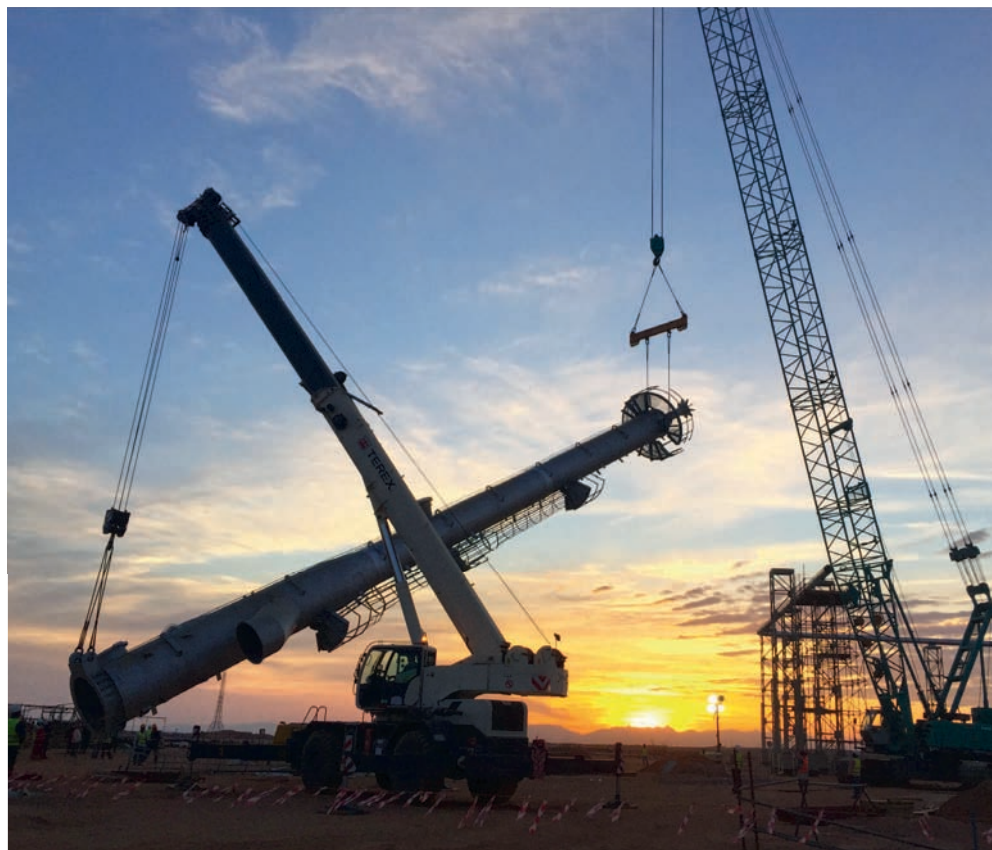
A crane works to erect a process flare stack at the Midyan gas plant project site. Started in 2013, construction on the plant is now more than 86% complete, and it is scheduled to go into full operation by the end of the year.
